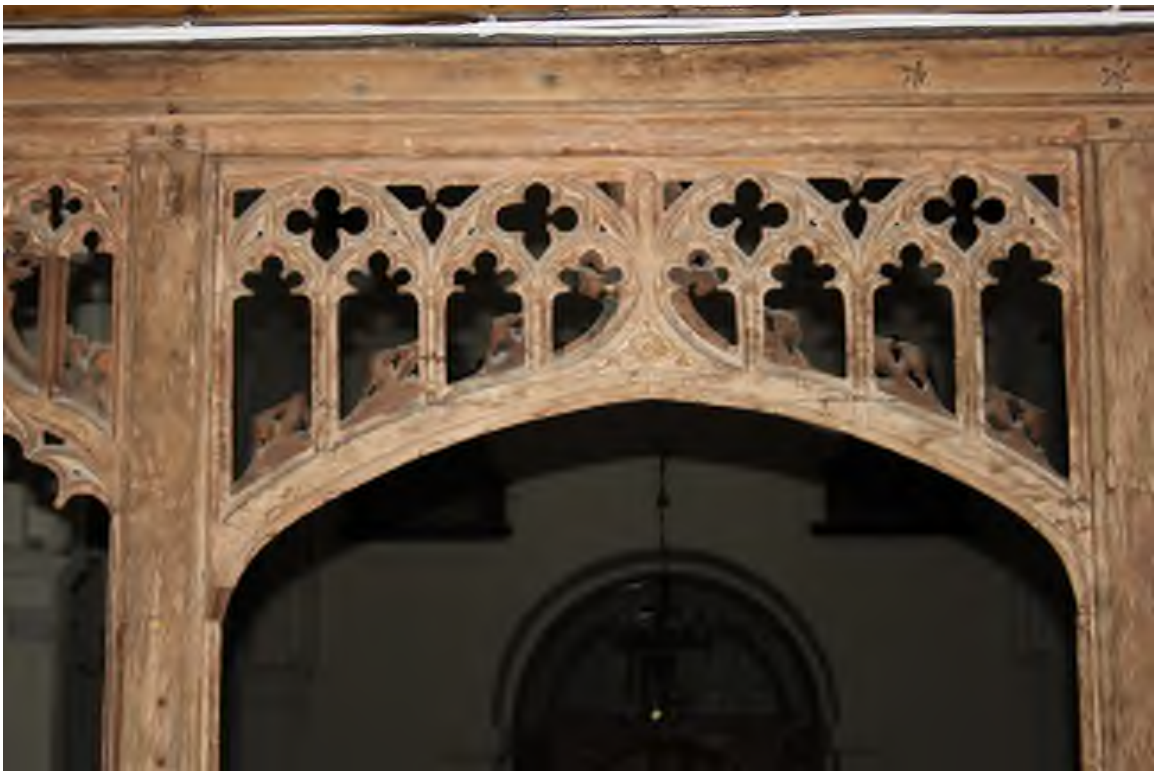
St Nicholas, Stevenage. Flat east face of rood-screen. Note survival of the lead stars below electrical cabling.
